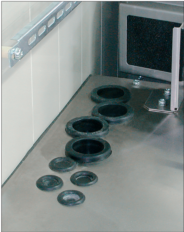
Cable entry made of rubber gland seals
