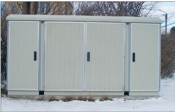
The cabinet after extension
